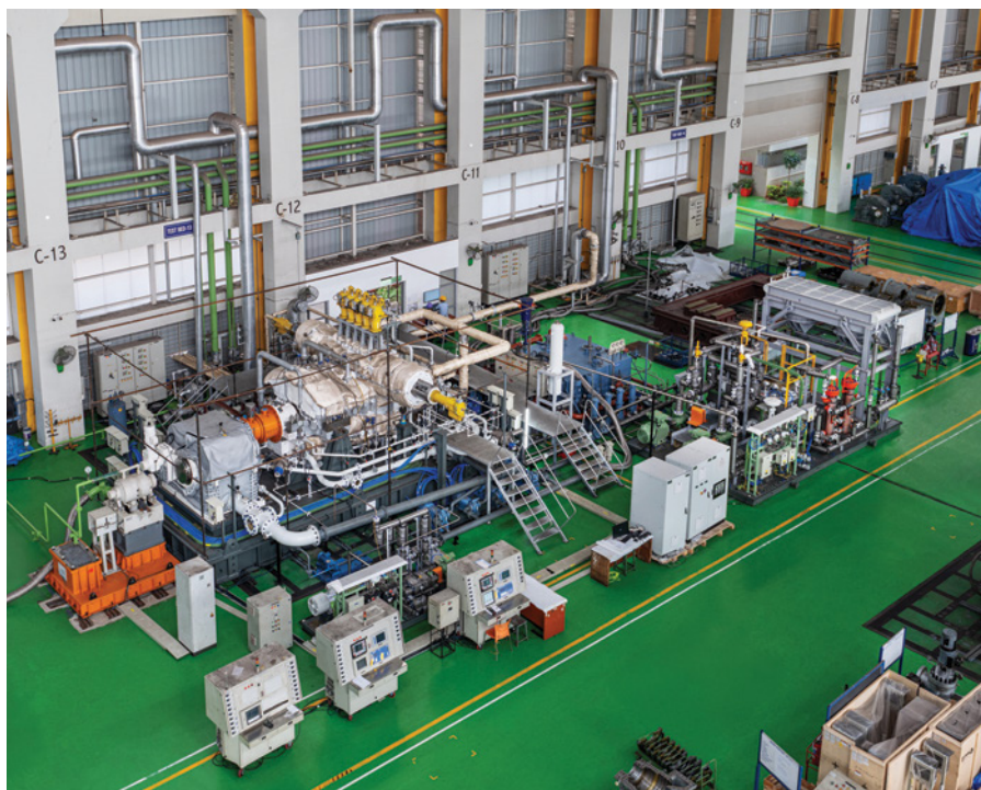
1. Steam turbine assembly and testing facility at Triveni Turbine's state-of-the-art manufacturing plant. Courtesy: Triveni Turbine Ltd.
