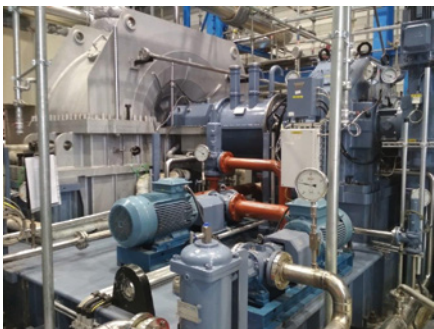
2. State-of-the-art WtE power plants utilize steam turbine generators to produce electricity. Courtesy: Triveni Turbines
