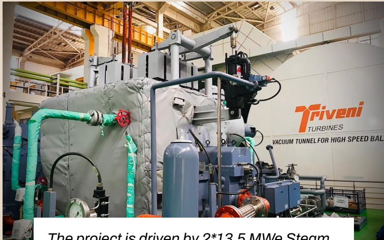
The project is driven by 2*13.5 MWe Steam Turbine installed in South Africa
