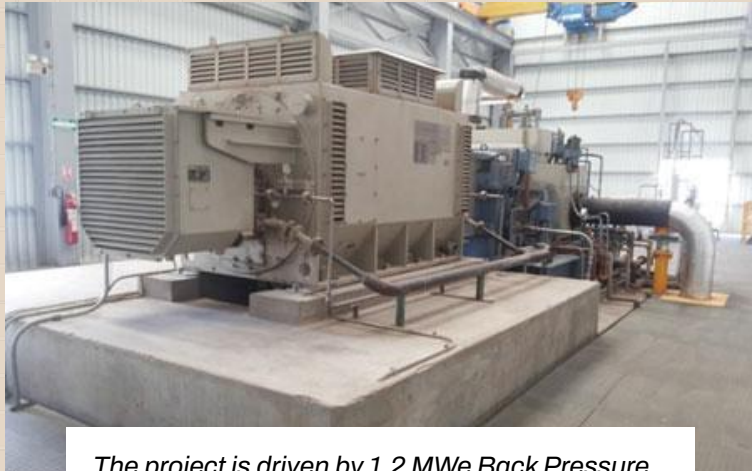
The project is driven by 1.2 MWe Back Pressure Single Stage Steam Turbine in Indonesia
