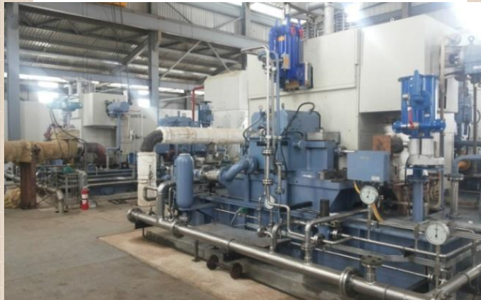
Bagasse-based cogeneration plant driven by 2*16.5 MWe straight back-pressure steam turbine with an inlet steam of 42 Bar and inlet temperature of 400 Deg C installed in Belize, Central America
