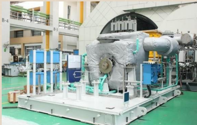
The project is driven by 1*3.6 MWe API 612 based Steam Turbine Generator cum Compressor Drive for an Oil Refinery in India
