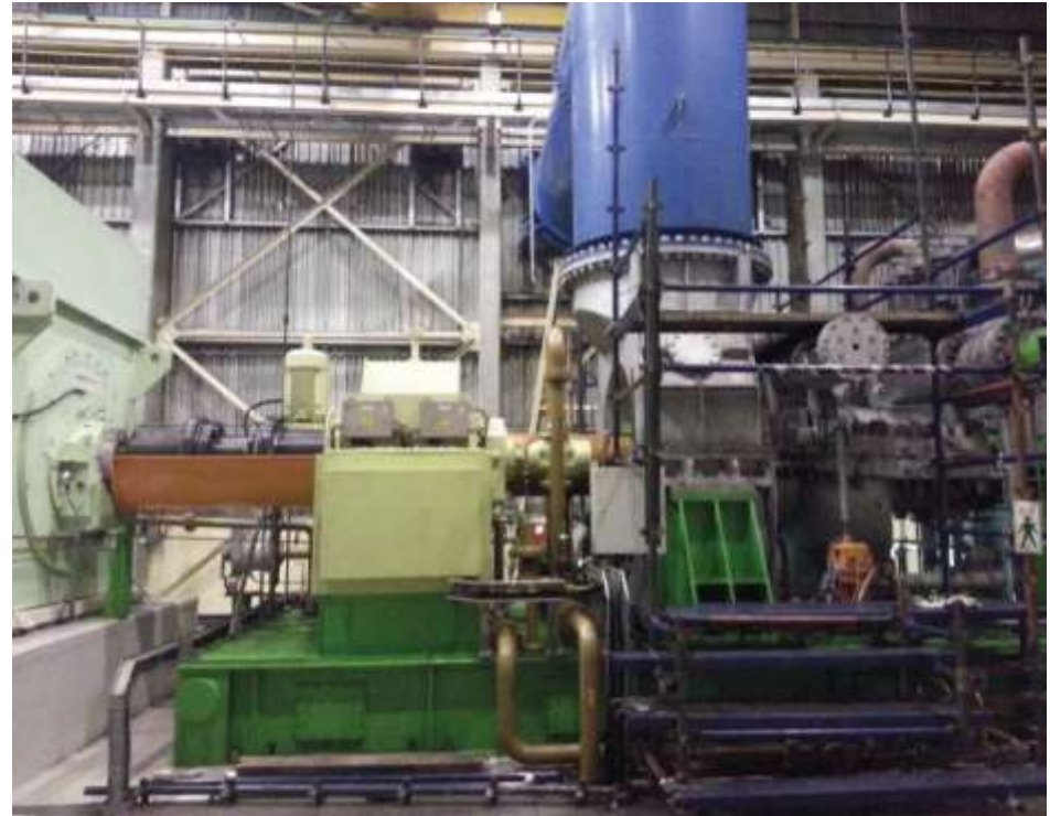
Plant after start up and synchronization
