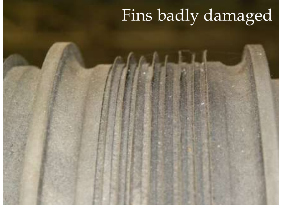
Blades damaged and corroded
